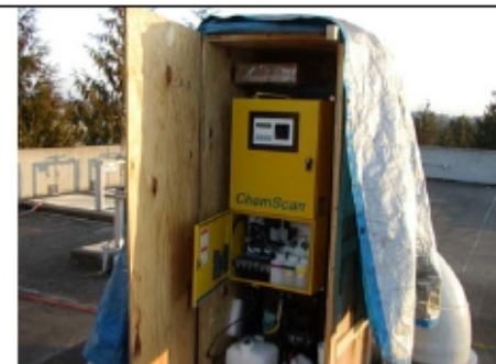
ChemScan System in Enclosure
