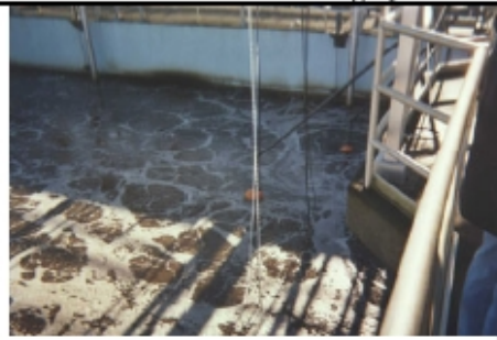
Danfoss Nitrate Monitors in Aerobic Zone
