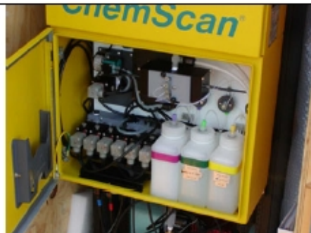
ChemScan System Internals
