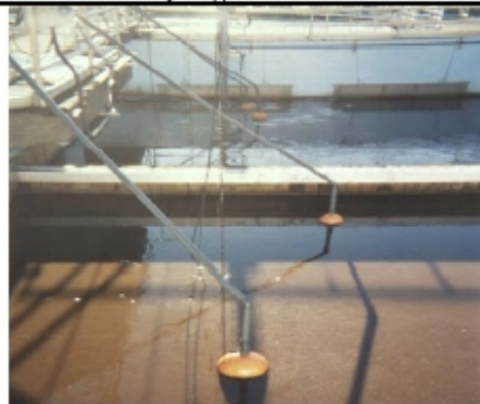
Danfoss Nitrate Monitors in Anaerobic and Anoxic Zones
